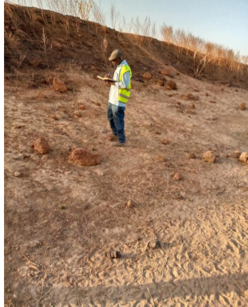
Downstream 1 in 2 not fully applied on embankment
