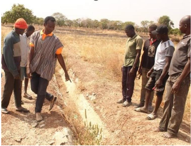
Plate 5. Breakages already at some portions of canals.
