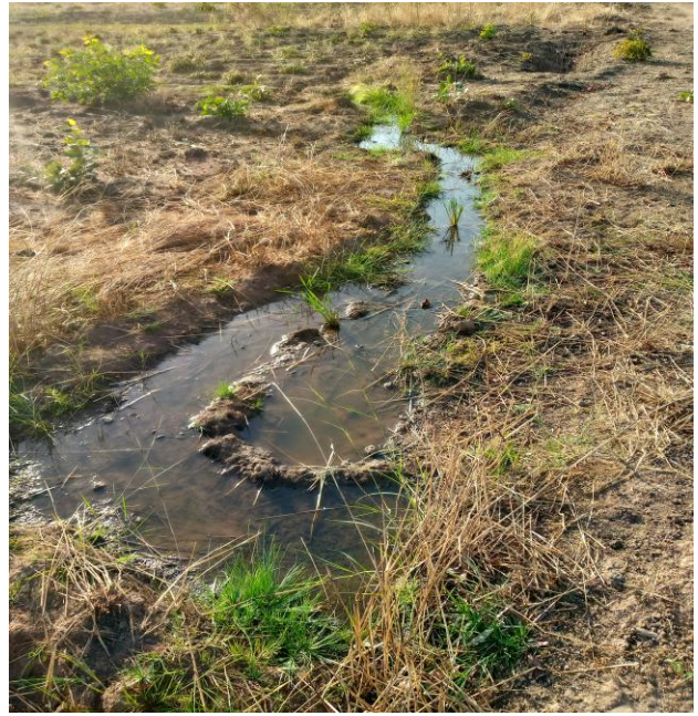
Plate 5b -leakages in the irrigable area along the main pipeline
